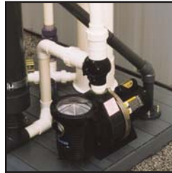
The HydraFin is plumbed and ready for installation
