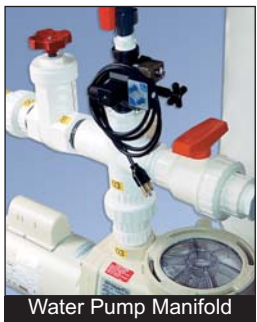
Water Pump Manifold
